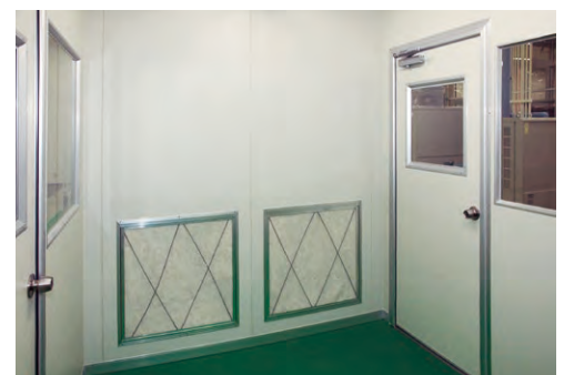
Example of External Air Intake
