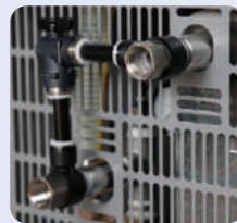
Chilled water flow and pressure controllers are indispensable.
