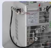
Can be used to monitor the chilled water circuit flow rate.
